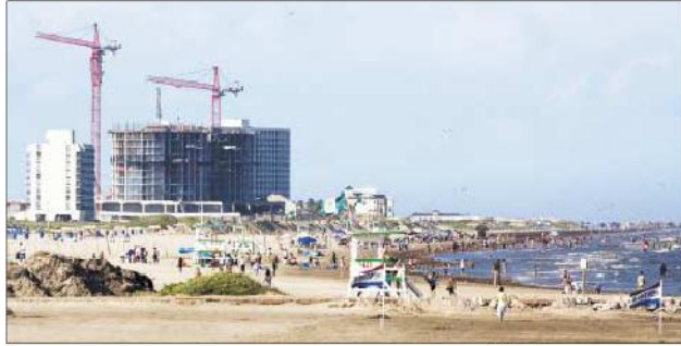
The twin 27-story towers of the Palisades Palms condominium project rise above Galveston's East Beach. How hot is the market here on the Gulf Coast? Of the project's 288 condos, 237 already are sold.
